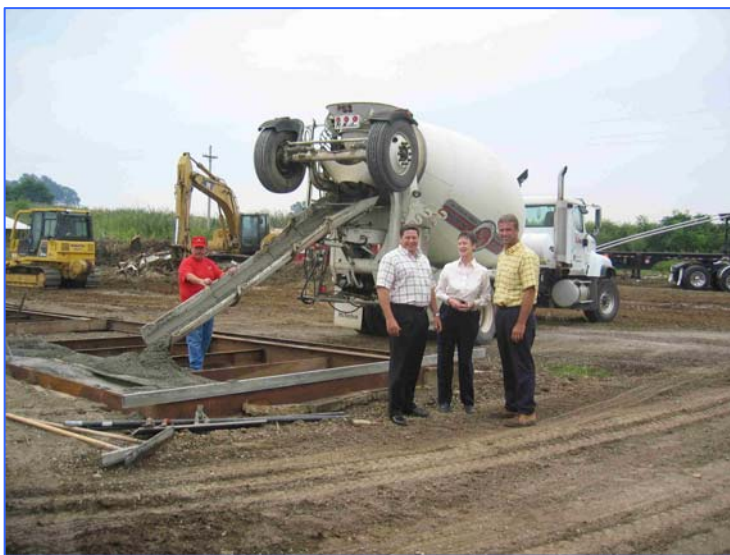
Martin Phillips, Marion Gilliland and Jeff Sidwell inspect the installation of concrete foundations.
